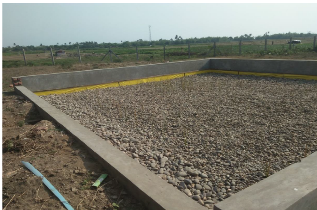
Figure 26: Secondary Constructed Wetland
