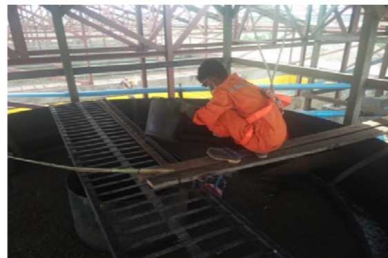
Figure 18: Scum Removal in HBT
