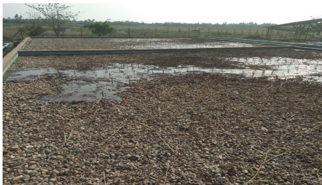
Figure 20: Constructed wetlands (The two beds run in parallel)
