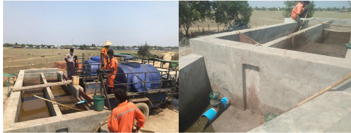
Figure 16: Emptying of tractors in the Dumping Station & Emptying of the reception tanks
